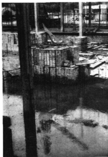
The hall at Sussex Way under construction — flooded even then —
